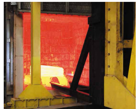
Batch Annealing Furnace
